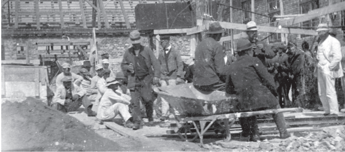
Arbejdere i færd med at udvide fabrikken op til jernbanestationen i Vester Aaby. Ca. 1920. DAMAS' arkiv. Workers busy with building the expansion of the factory up to the railway station in Vester Aaby. Approx. 1920. DAMAS archives.
